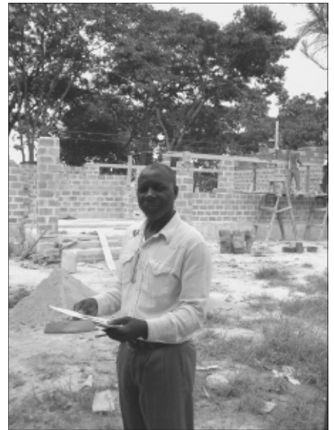
The new headmaster Hanyama Hakanyama supervising the construction of the new classroom block
